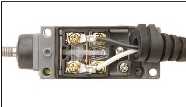
Figure 88. Belt tension limit switch wiring.
